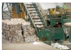
Solid waste compressor
